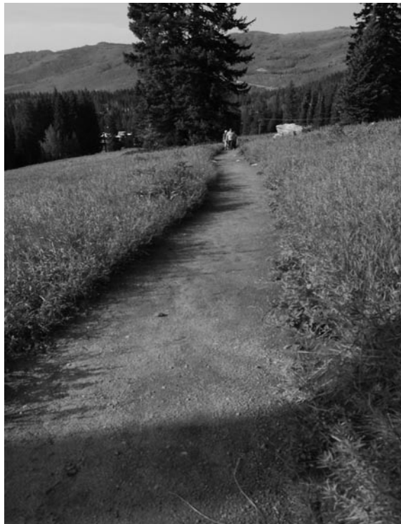
The new Lake Mary trail was dug by a trail building machine. It is wide enough to accommodate three individuals walking abreast.
